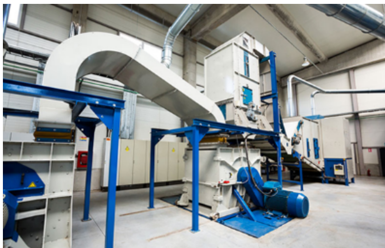
Figure 18: The wood separation unit of the fiber pulping plant of HempFlax Group B.V. in Oude Pekela (NL). Photo by the company
